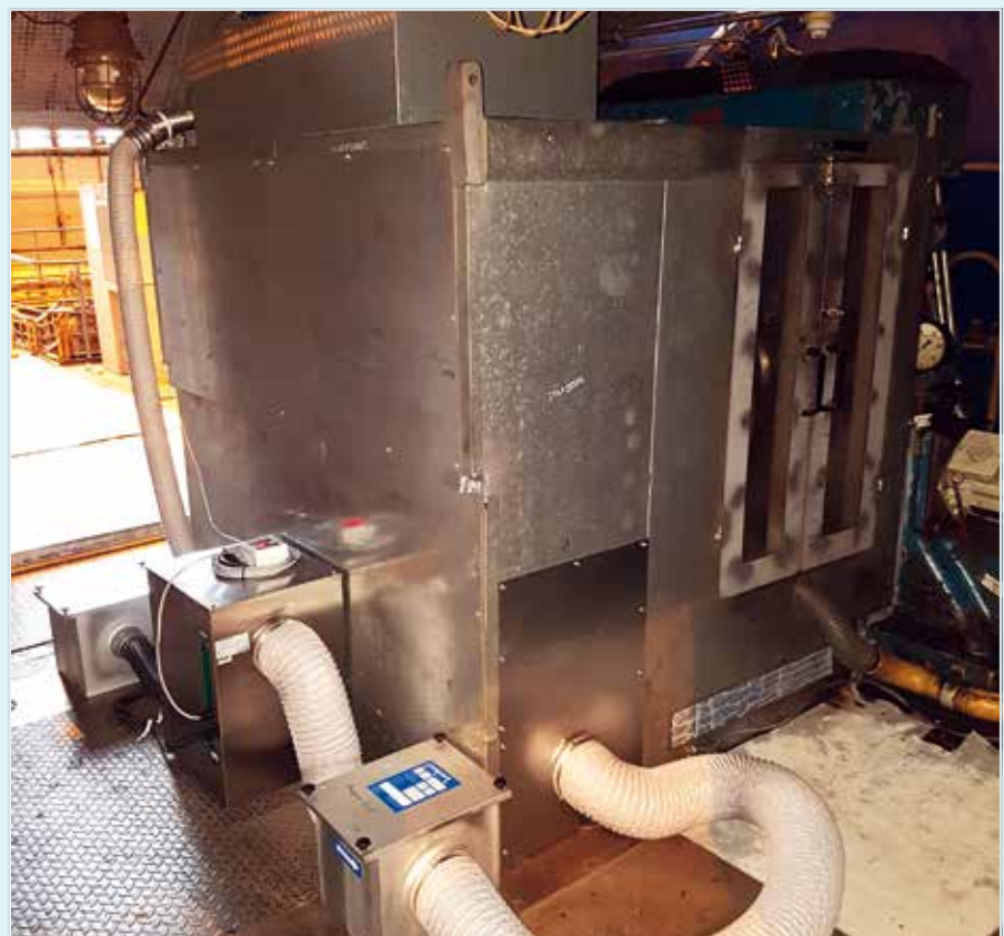
Abb. 2 Adsorptionstrockner Bürstenapparat Generator
